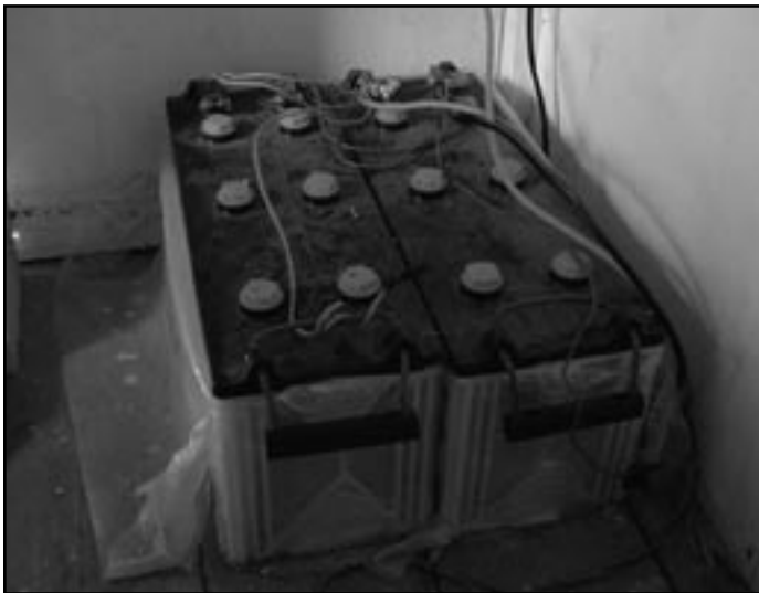
ABOVE: Computers are powered by batteries that are recharged daily using solar panels.
